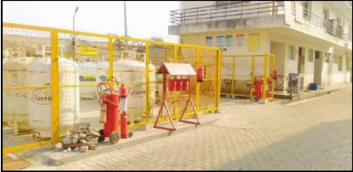
Photographs showing Fire Safety Equipment
