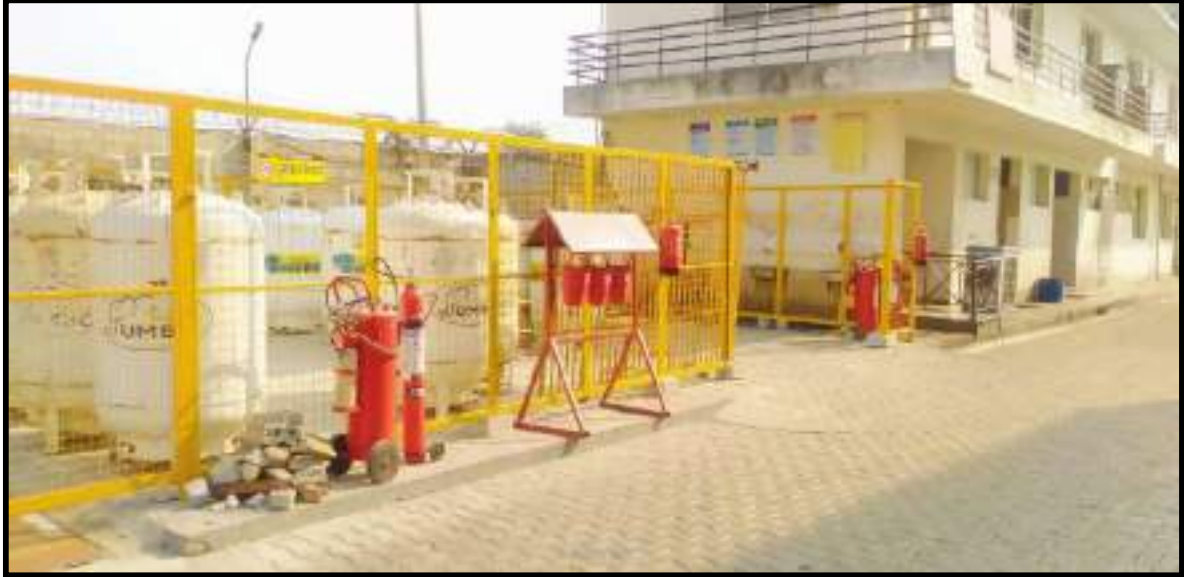
Photographs showing Fire Safety Equipment
