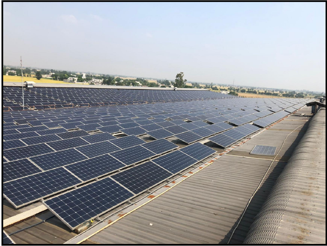
Photographs showing Solar Panels
