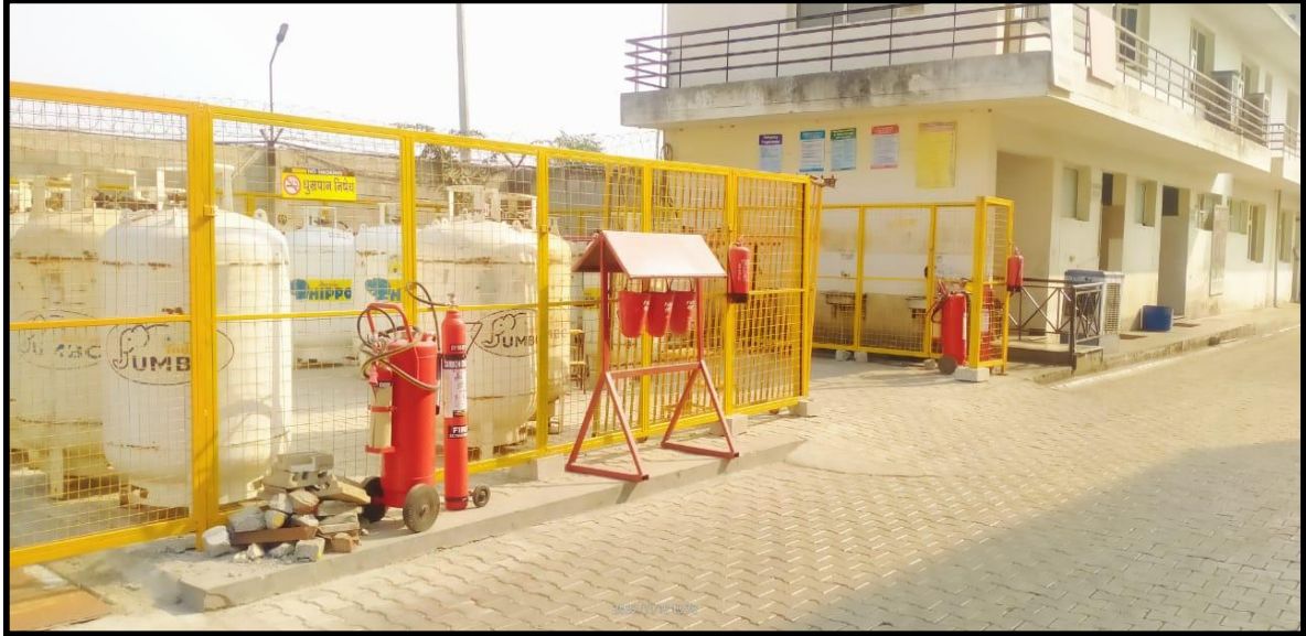
Photographs showing Fire Safety Equipment
