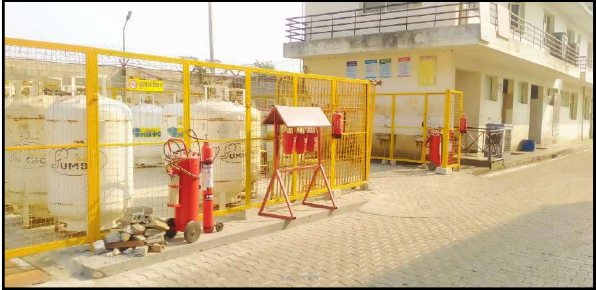
Photographs showing Fire Safety Equipment
