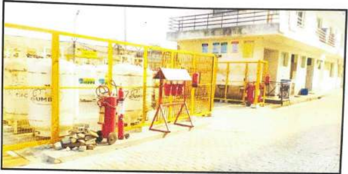
Photographs showing Fire Safety Equipment
