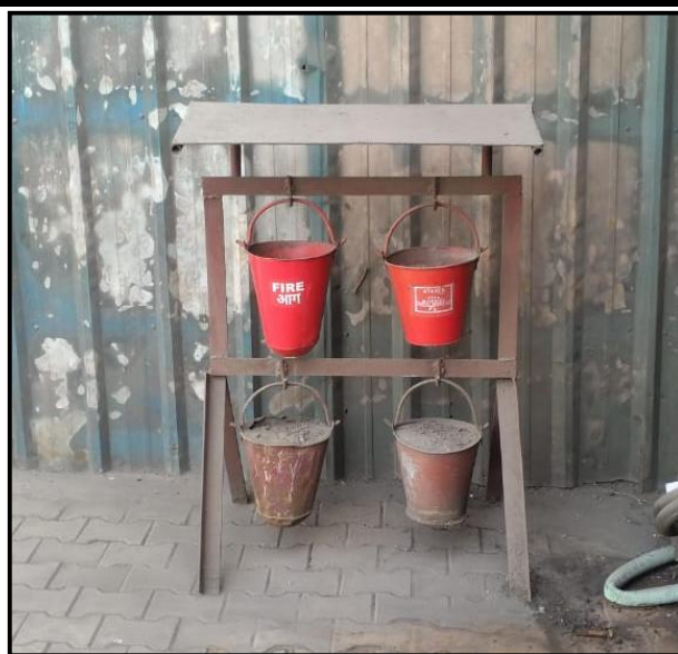
Photographs showing Fire Safety Equipment
