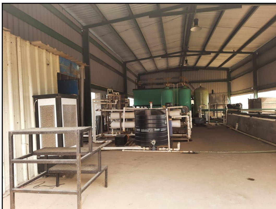
Photographs showing Effluent Treatment Plant
