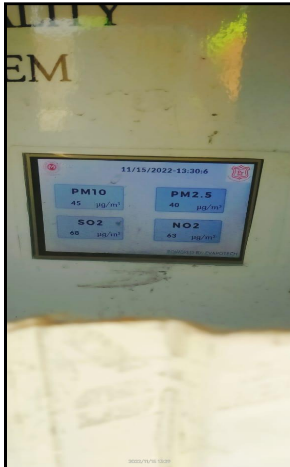
Photograph showing Ambient Air Monitoring System installed
